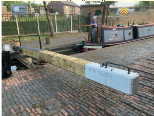
The new top gate at Wolverhampton Top Lock; just four days after installation.
